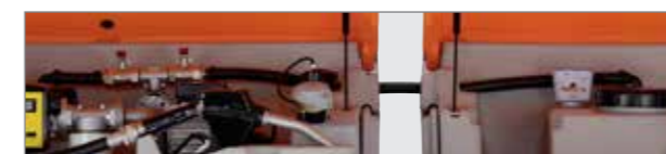
Delivery line with connection to first tank and switching valves included in scope of delivery of the expansion unit.
